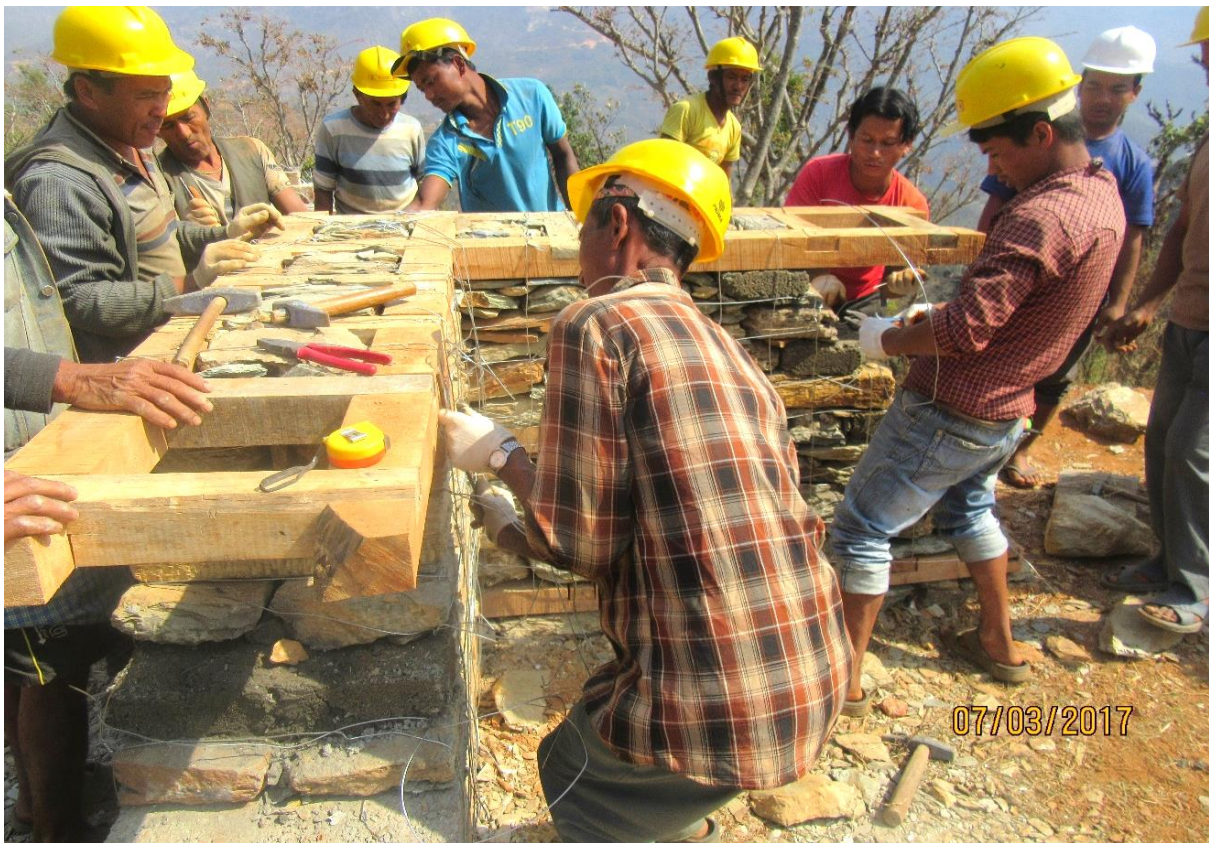
Participants working on construction of wooden bands during hands on practical exercise of rural mason training in Dhading
