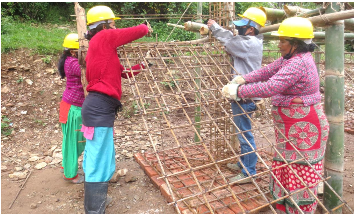
Figure 7. Participants, including female masons working on construction of reinforcement frame of staircase during urban mason training in Bhimeswar, Dolakha. Although female masons are quite few in number, Baliyo Ghar Program made considerations to ensure their inclusion as much as possible.
