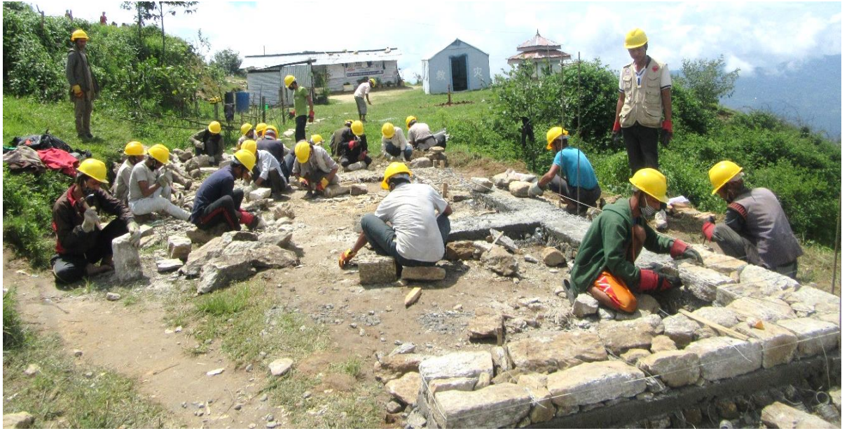
Figure 3. Training participants working together in construction of stone masonry walls using earthquake resistant construction techniques in Dolakha. Participants constructed a small scale model of masonry walls to apply hands on practice of the techniques of construction under close supervision of instructors.
