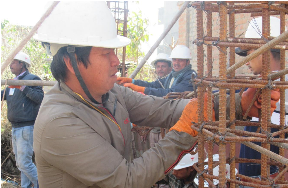
Figure 11. A group of participating masons try hands-on exercise in rebar placement and binding to construct RC frame columns and beams during urban mason training in Kathmandu.
