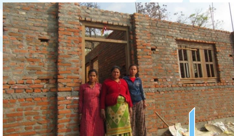
Mrs. Sabitri with her daughters in front of her under construction home
