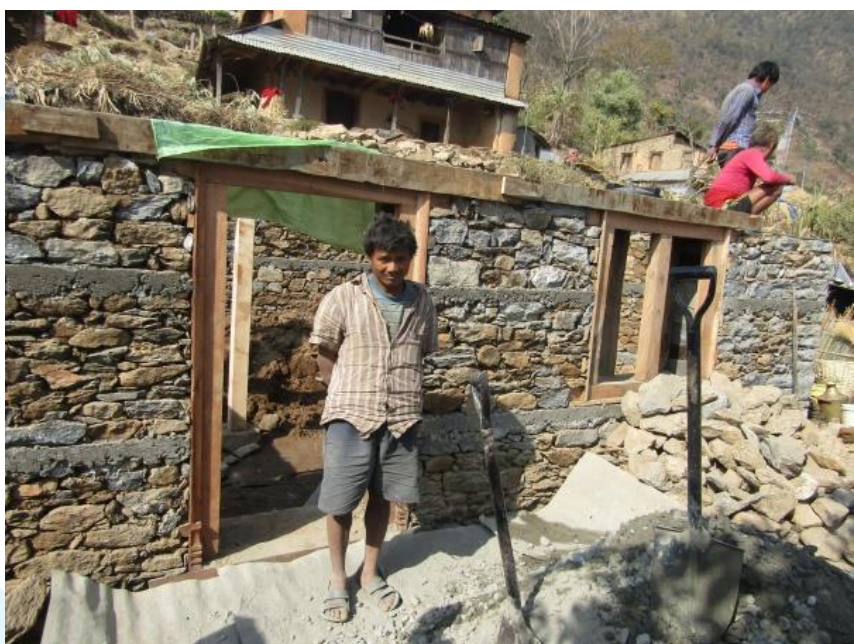
Mason Mr. Bir Bahadur Tamang in front of a house he build recently
