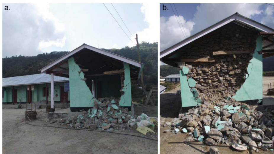
Figure 1. Damaged building of Sumnima Pre-secondary School in Panchthar district of Eastern Nepal after the Sikkim/Nepal border earthquake of September 18, 2011. More damage was noticed in the recently constructed building.
