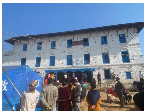
Service receivers at CDO office with damaged Durbar in the background
