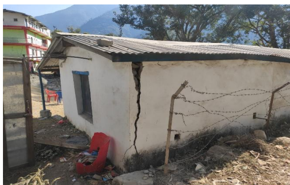
Structural damages observed and documented during assessment at Nalgadh Municipality
