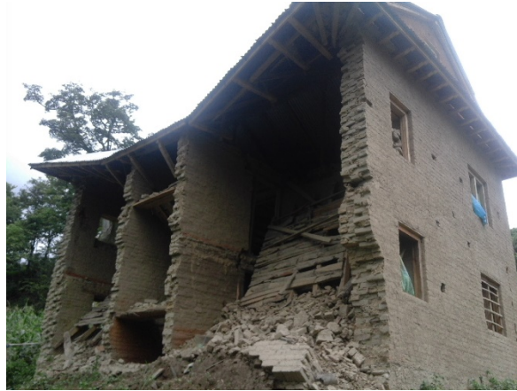
Figure 2: A rural building damaged by the Gorkha Earthquake.
